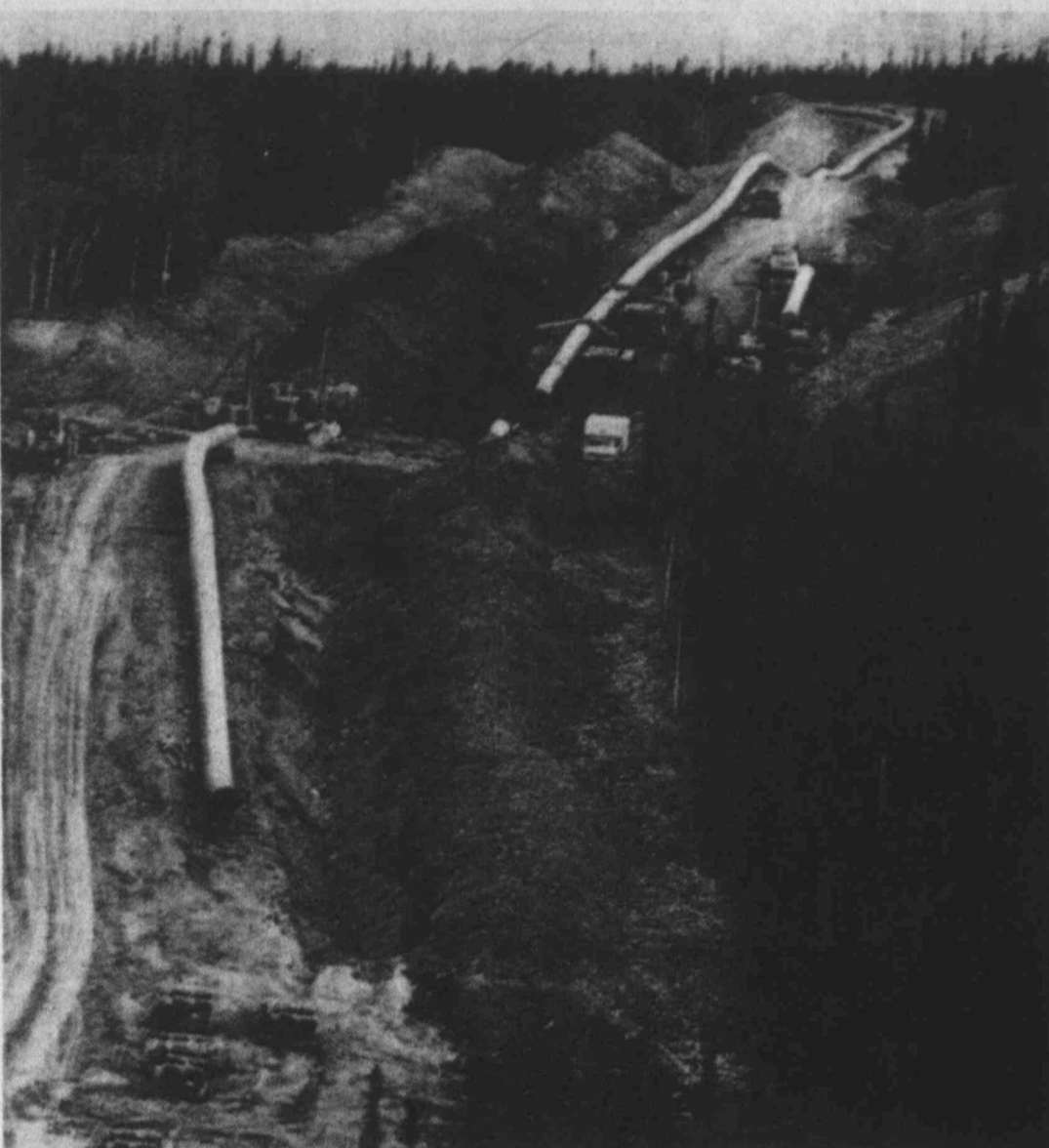
COMING OVER THE HILLS — A string of 48-inch-diameter pipe for the trans-Alaska pipeline is readied for burial in a hilly area about 10 miles north of the Yukon River. The 800-mile-long pipeline is scheduled to begin pumping oil from Alaska's Prudhoe Bay to Valdez in 1977.
