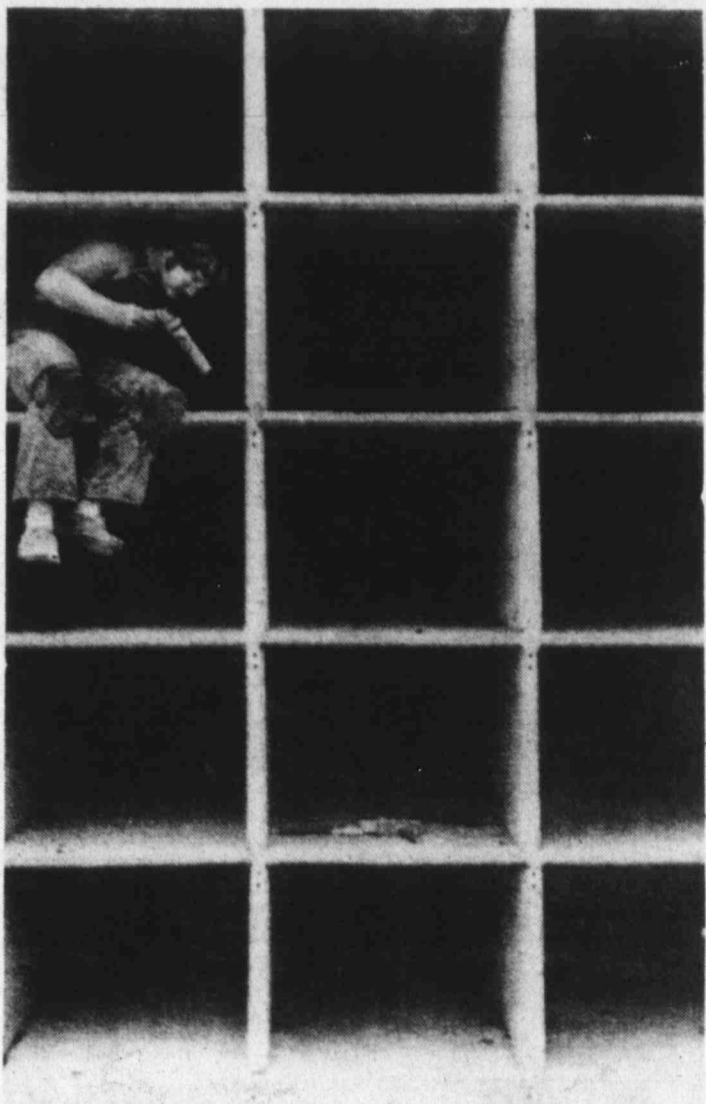
CAULKING A CUBICLE — Mike Sewell found that strapping rubber soles of shoes to his knees eased the wear-and-tear as he caulked a cubicle in a mausoleum under construction at Resthaven Memorial Park in Louisville, Ky.
