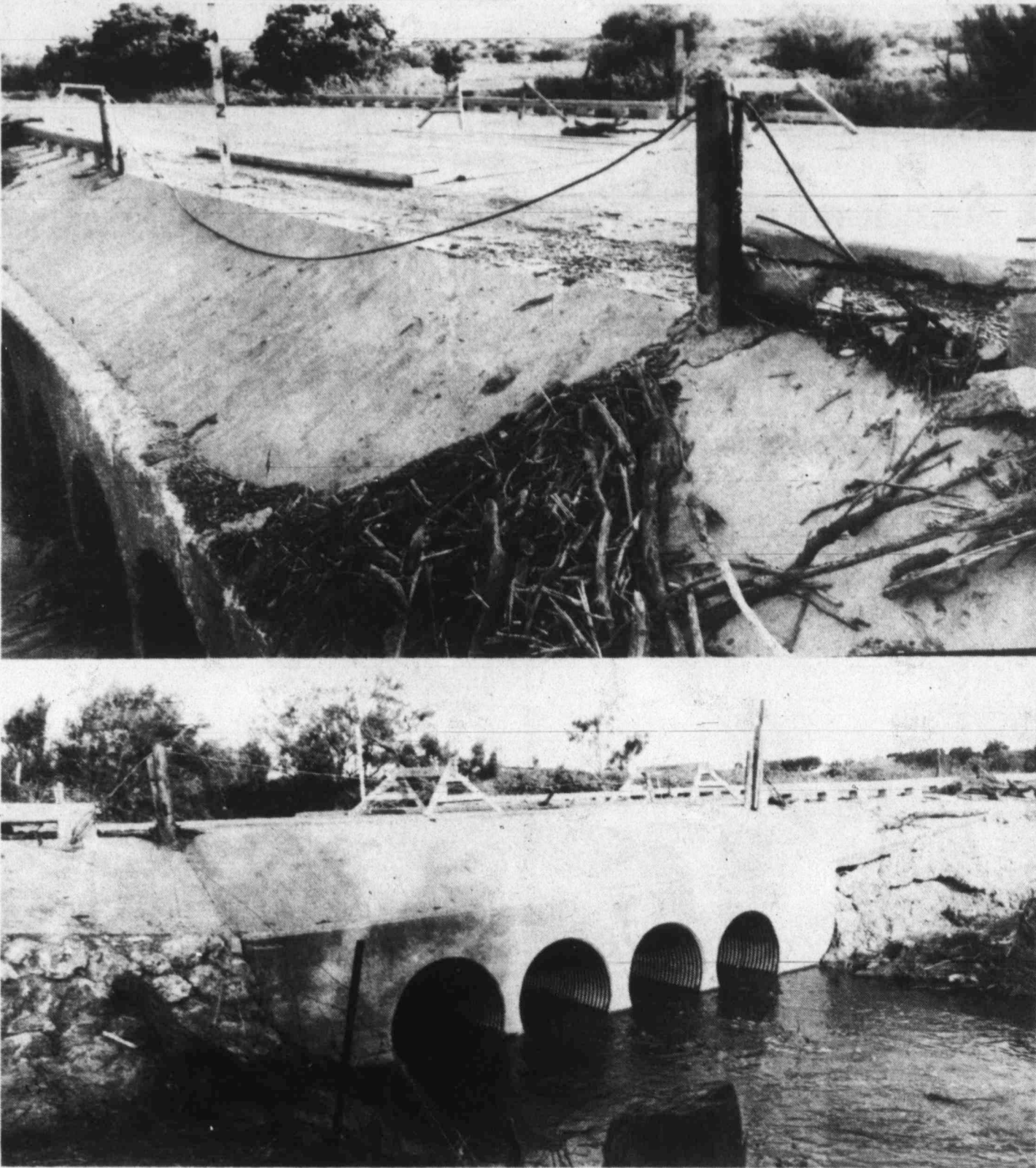
BRIDGE CAVES IN — The bridge on the only road to Moss Creek Lake collapsed in one lane, and County Commissioners Court Thursday afternoon authorized emergency repairs. Recent rains washed out soil supporting the bridge already weakened by acid but treated sewer water, County Engineer Neel Barnaby said.
