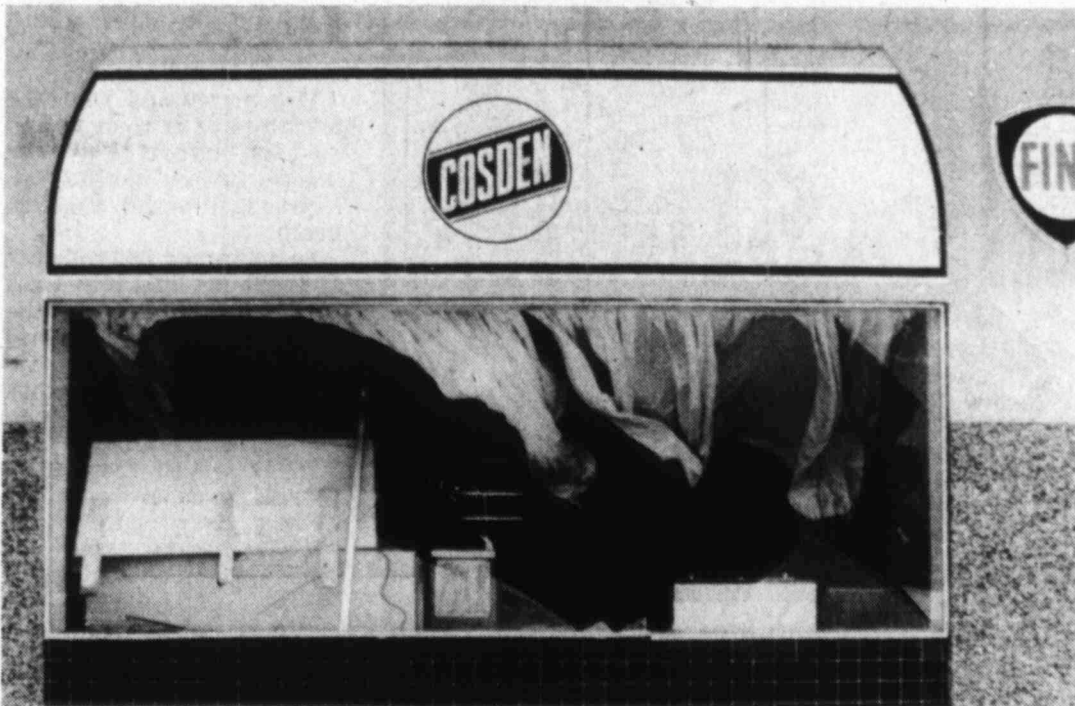
ONE INJURED — Neil Ray McCrary was cut on the feet and legs when a window blew in at 12:55 p.m. today in the snack bar area at the west end of the Cosden Office building. Winds were reported to be up to 35 miles per hour when a cold front hit shortly before noon. Mrs. McCrary was hospitalized at Medical Arts.
