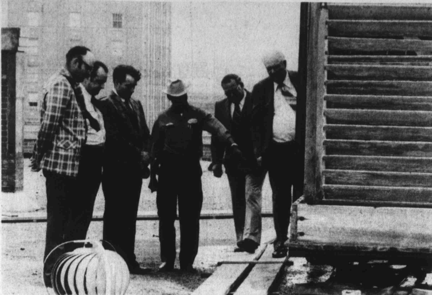
HIGH-LEVEL DISCUSSIONS — Members of County Commissioners Court look over a leaking cooling tower on the courthouse roof. Pointing out the problem is Eddie Harper, building maintenance supervisor. From left to right are Commissioners Jack Buchanan, William B. Crooker Jr. and Ikie Rupard, Harper, County Judge Bill Tune and Commissioner Simon (Cy) Terrazas.
