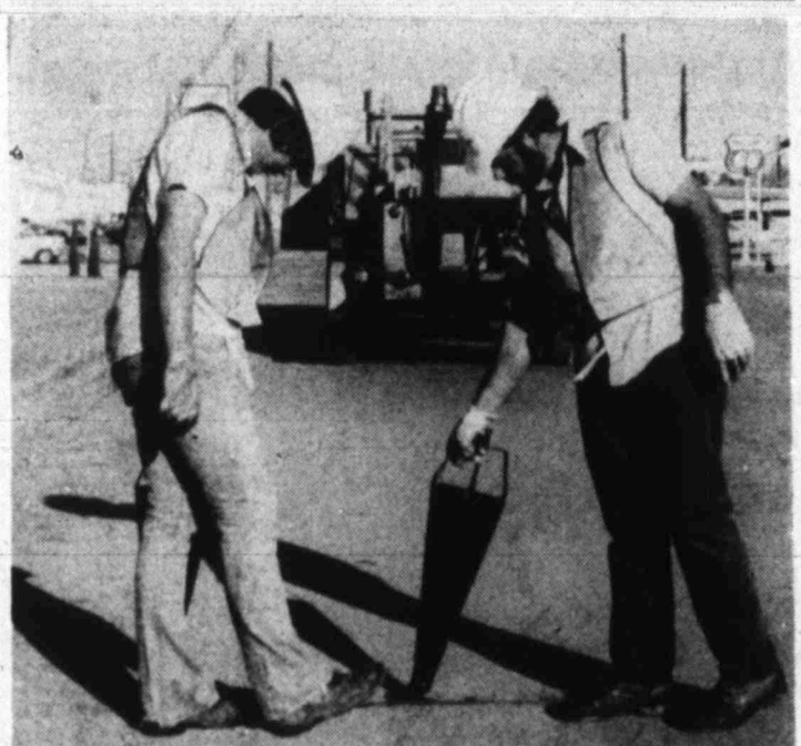
SEALING CRACKS IN STREET — Texas Highway Department workers seal cracks on Fourth Street with hot asphalt. During good weather, THD men are doing this kind of work on state roads all over Howard County, Darwin D. Webb, THD county maintenance foreman, said. Also, the department is winterizing some farm roads with an emulsion of water and asphalt, Webb said. Working here are (left to right) Bill Lewis and Joe Del Bosque. Robert Rodriguez was manning the truck.
