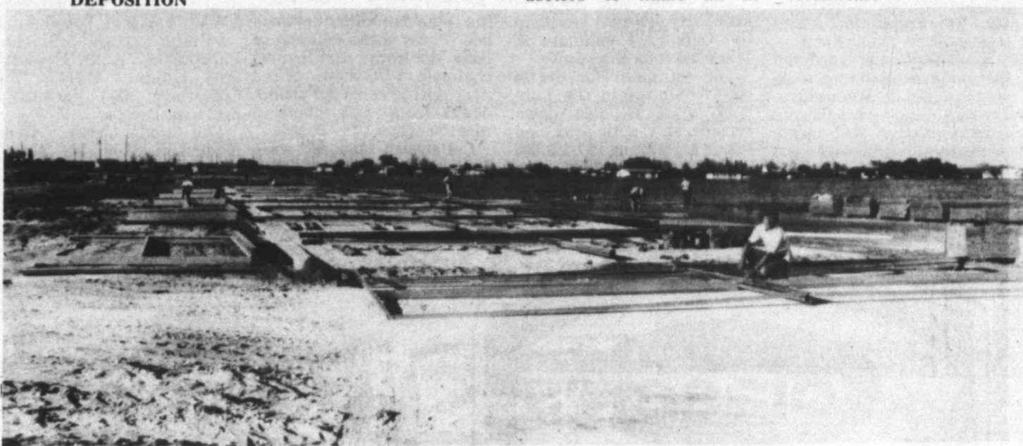
DUE TO BE COMPLETED — Workers lay steel beams for 10 additional hangers at Howard County Airport. Chaparral Contractors has promised to complete the structures before the end of November, weather per-
