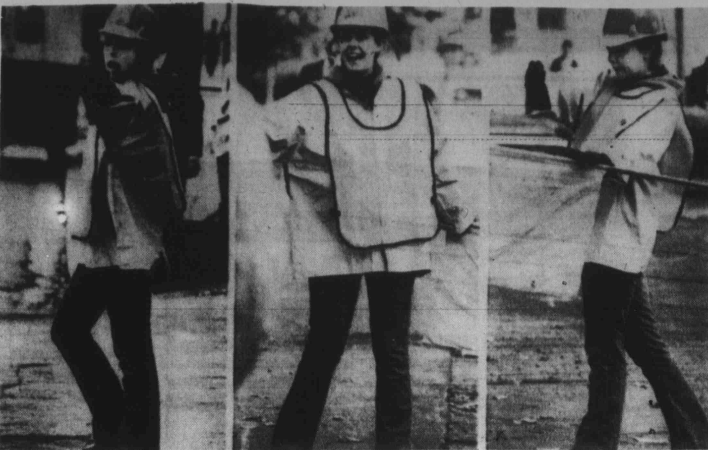
BODY ENGLISH — Debora Workinger, 21, of Falls Church, Va., shows a variety of traffic direction signals as she works on a Washington construction site. Miss Workinger says that, while she may "swear a lot," she does not really get angry at motorists and enjoys the work except for her 6:30 a.m. starting time. When she is not detailed to traffic direction, she works as a laborer pouring concrete.
