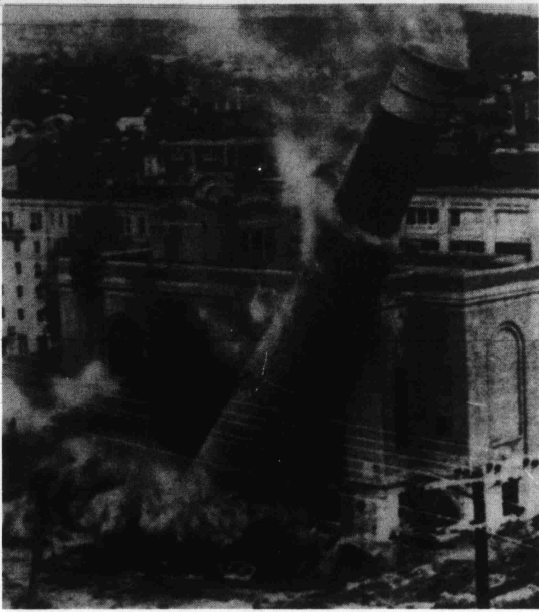
LEANING TOWER OF BRISTOL — A 210-foot smokestack at the New Departure Co. power plant topples Sunday morning in Bristol, Conn., after workers set off explosives to bring it down. The tower was removed as part of a redevelopment project.
