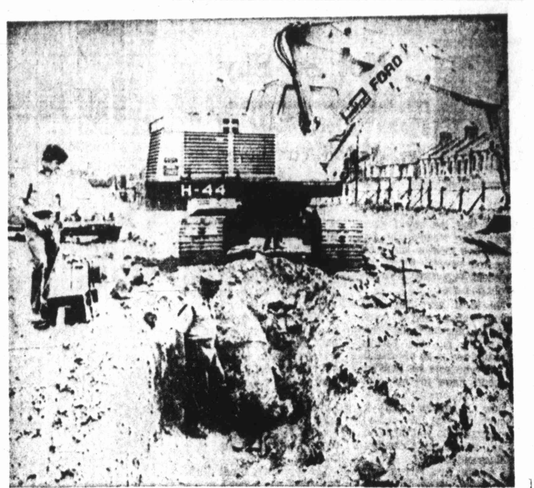
WARTIME BOMB UNEARTHED — Maj. Arthur Hogben, in hole, of the 49th Explosive Ordnance Disposal Unit, Royal Engineers, and Karl Bradbury, of Marazion, Cornwall, check World War II bomb unearthed Thursday at a building site in East London. Authorities said bomb was dropped by the German Luftwaffe in an air raid on the British capital. At least 1,000 people were evacuated from their homes while experts deal with the bomb.
