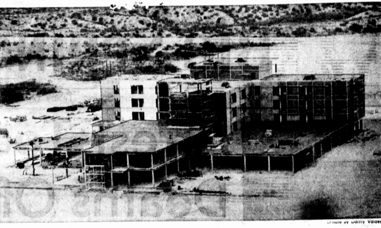
TAKING SHAPE — The new HCA hospital plant is taking shape on the tract below Scenic Mountain. Exterior walls are mostly in place and the impregnation of the white marble aggregate will take place soon (as in panel at left). The 150-bed structure, with service core designed to carry twice that number of beds, is running well ahead of schedule.
