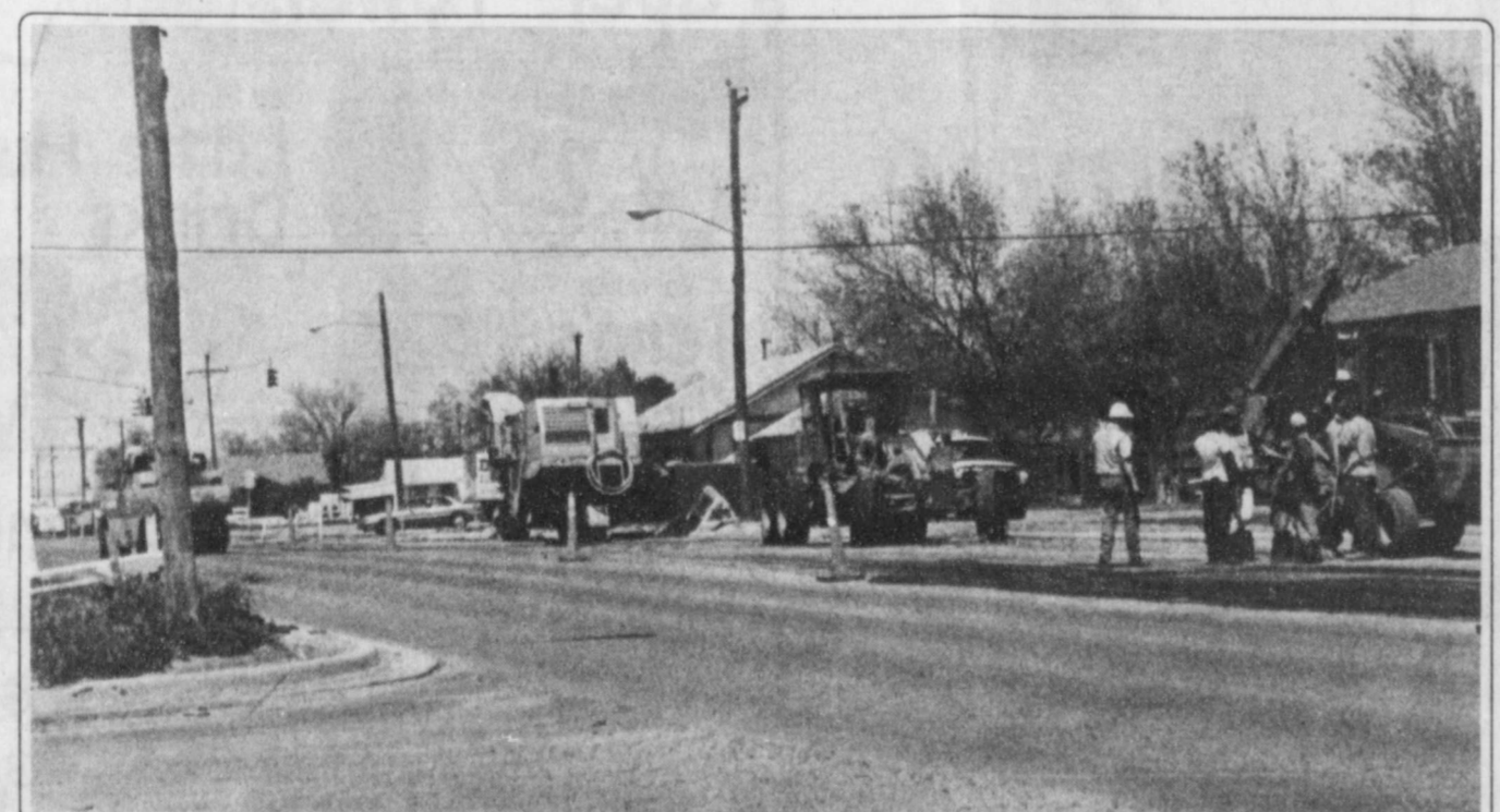
ROAD CONSTRUCTION MOVING AHEAD AGAIN-- Pretty weather has allowed the construction crews to get back to finishing their paving on Second Street in Floydada. Mike Anderson of the Floyd County Highway Maintenance Department said, "The city has raised some of their manhole covers and the driveways and sidewalks are being poured on Houston Street. A final 1 1/2 inch hot mix topping will be added to the streets under repairs when everything else is finished." Staff Photo
