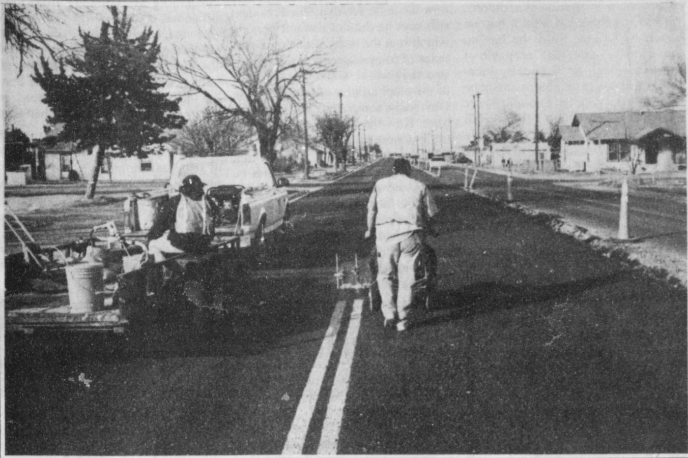
OPENING SOON--Highway workers on 2nd Street in Floydada place striping on a new section of road. This week, the west side of 2nd Street (Hwy. 70) will be open through town and then construction will start on the east side of the road.
