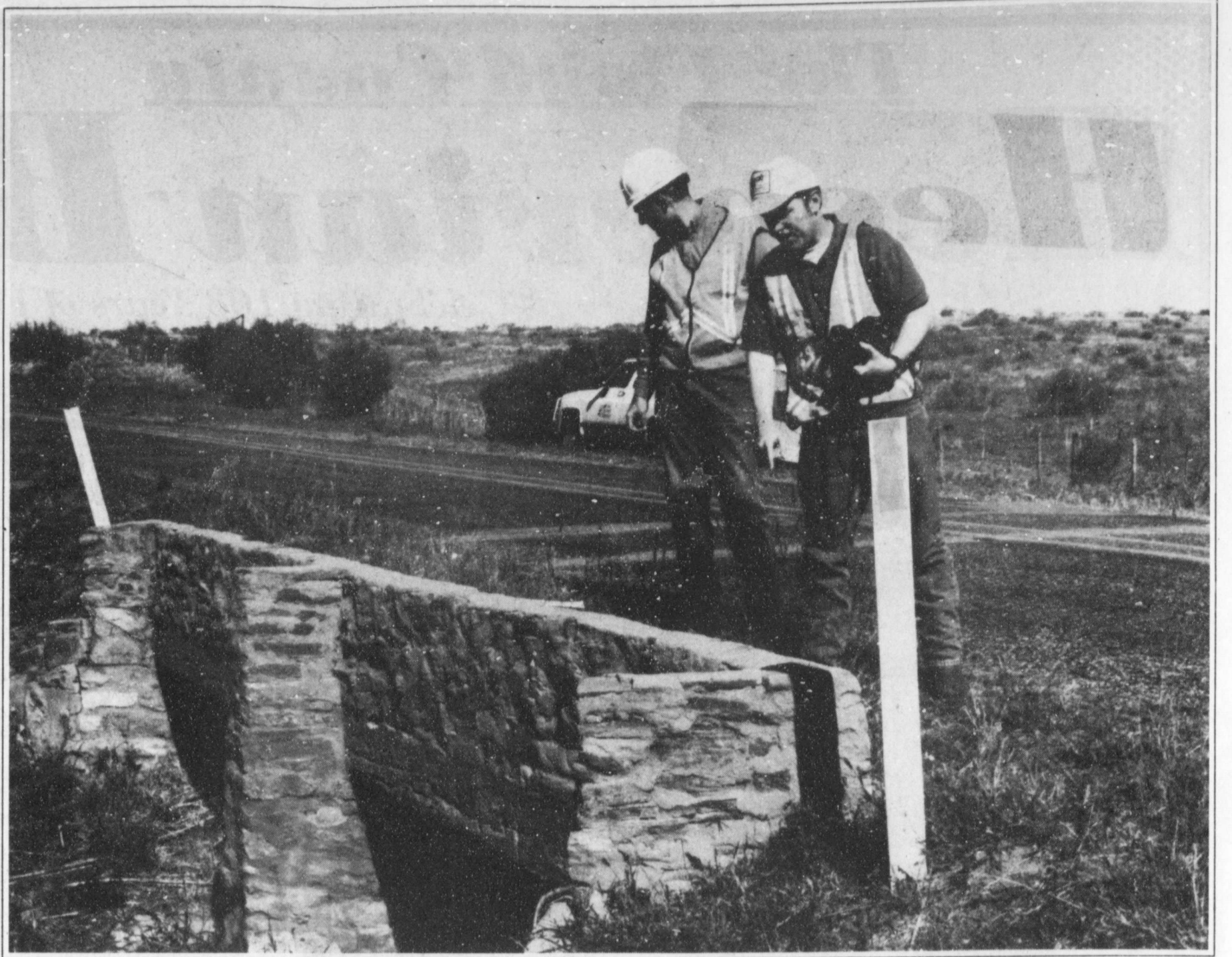
Matt Evans, Lubbock District Environmental Coordinator (left) and Rick Mitchell, Austin Division historic preservation planner (right), inspect a masonry bridge on FM 1065 in Floyd County. The bridge is the last one
