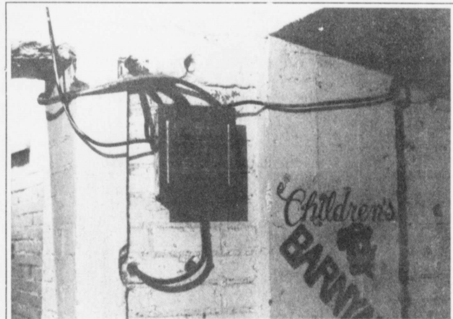
FAIR WIRING --This picture is a good example of the wiring that Fair officials, and vendors contend with in the of Fair Building in Lockney.
