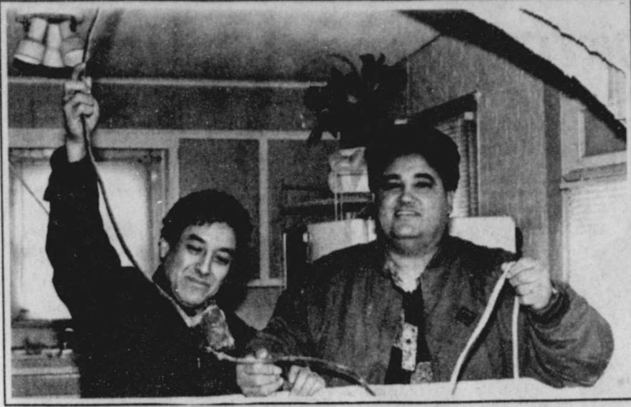
CHURCH MEMBERS AT WORK--Gabriel Padilla Sr. and Rev. Juan Gutierrez work on wiring after arched window is cut between kitchen and future serving area. Staff Photo
