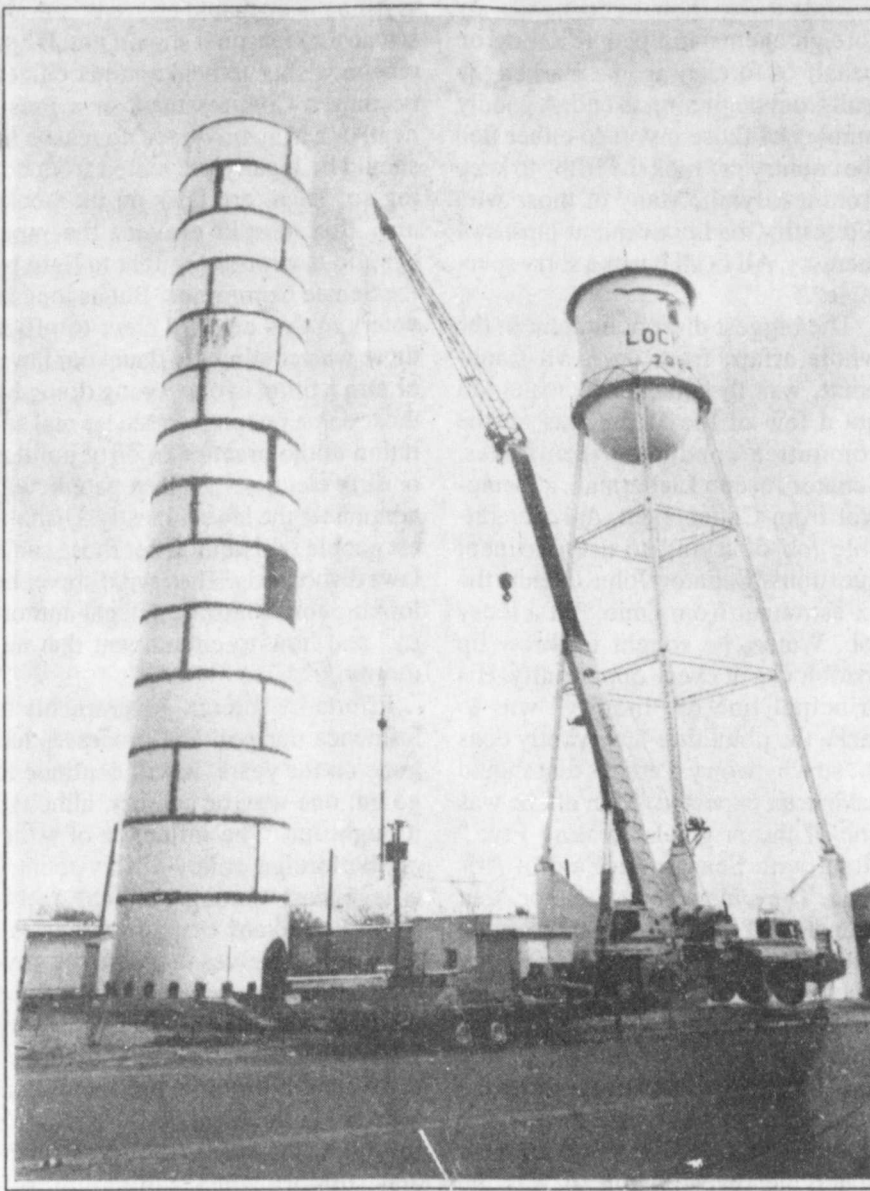
A NEW LOOK--The new water tower in Lockney has a different appearance than Lockney's familiar landmark water tower. Nearing completion the new tower is ground based with no support legs and resembles a huge grain silo. According to City records the first water storage facility was erected in 1917. According to Utilities Superintendent Dickie McCarty the new facility is replacing the tower which was built in 1929. Staff Photo
