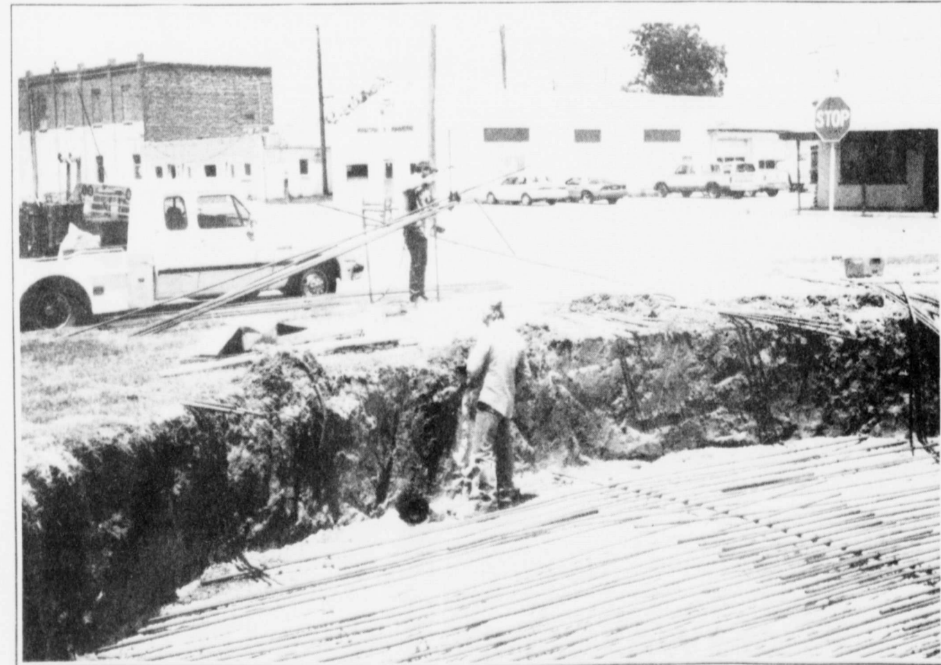
WATER TOWER CONSTRUCTION BEGINS-- The City of Lockney has begun construction on a new water tower. The tower, which is scheduled to be finished
