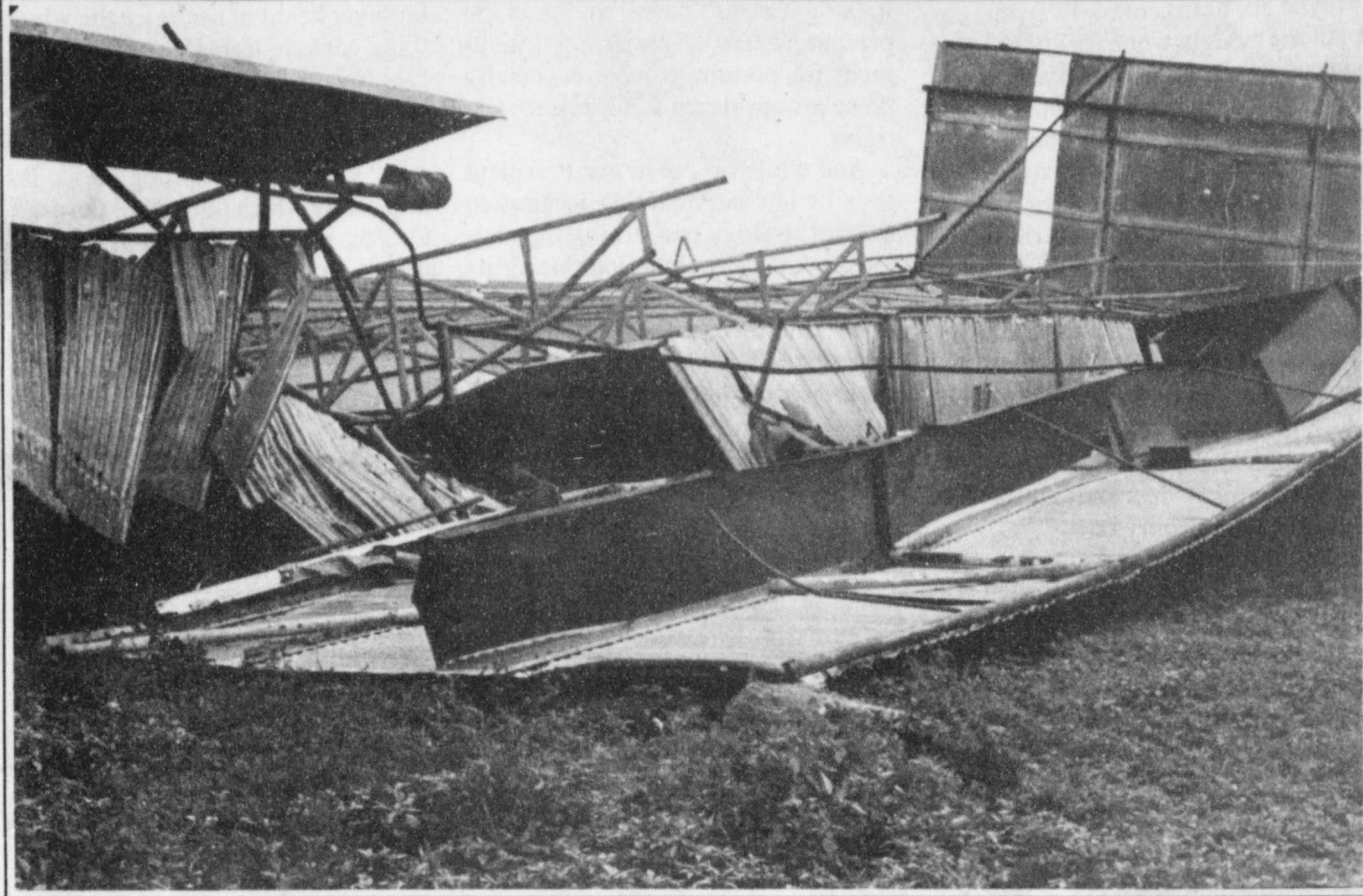
BARN SCRAPS --The barn, belonging to Jack Miller, north of Floydada, was turned upside down by Saturday afternoon's winds. The barn was enclosed except for the south side. Staff Photo
