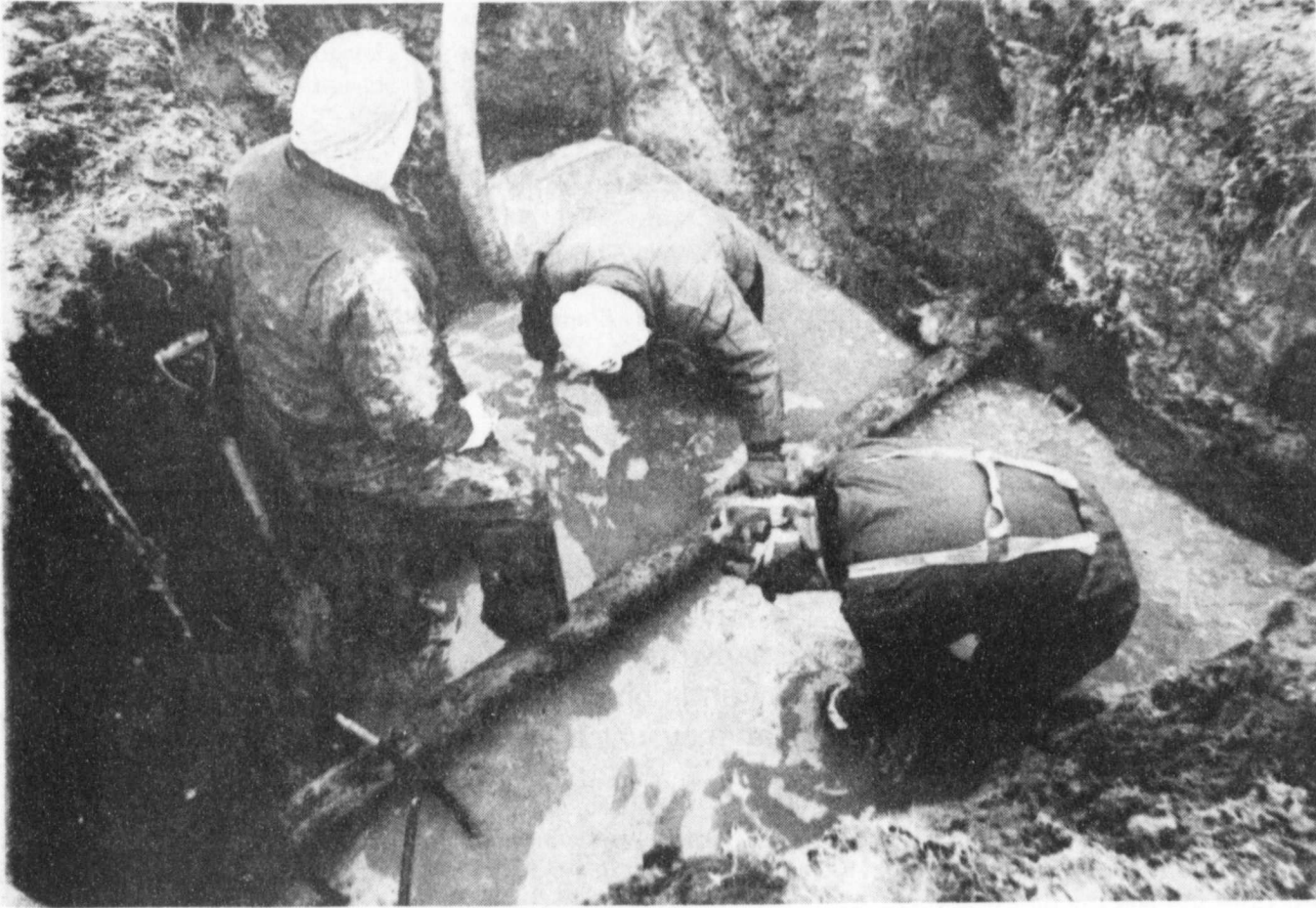
WINTER HAZARDS --Freezing temperatures and a broken water main created terrible working conditions for Floydada workers as they battled temperatures of 15 degrees and below and the chilling water
