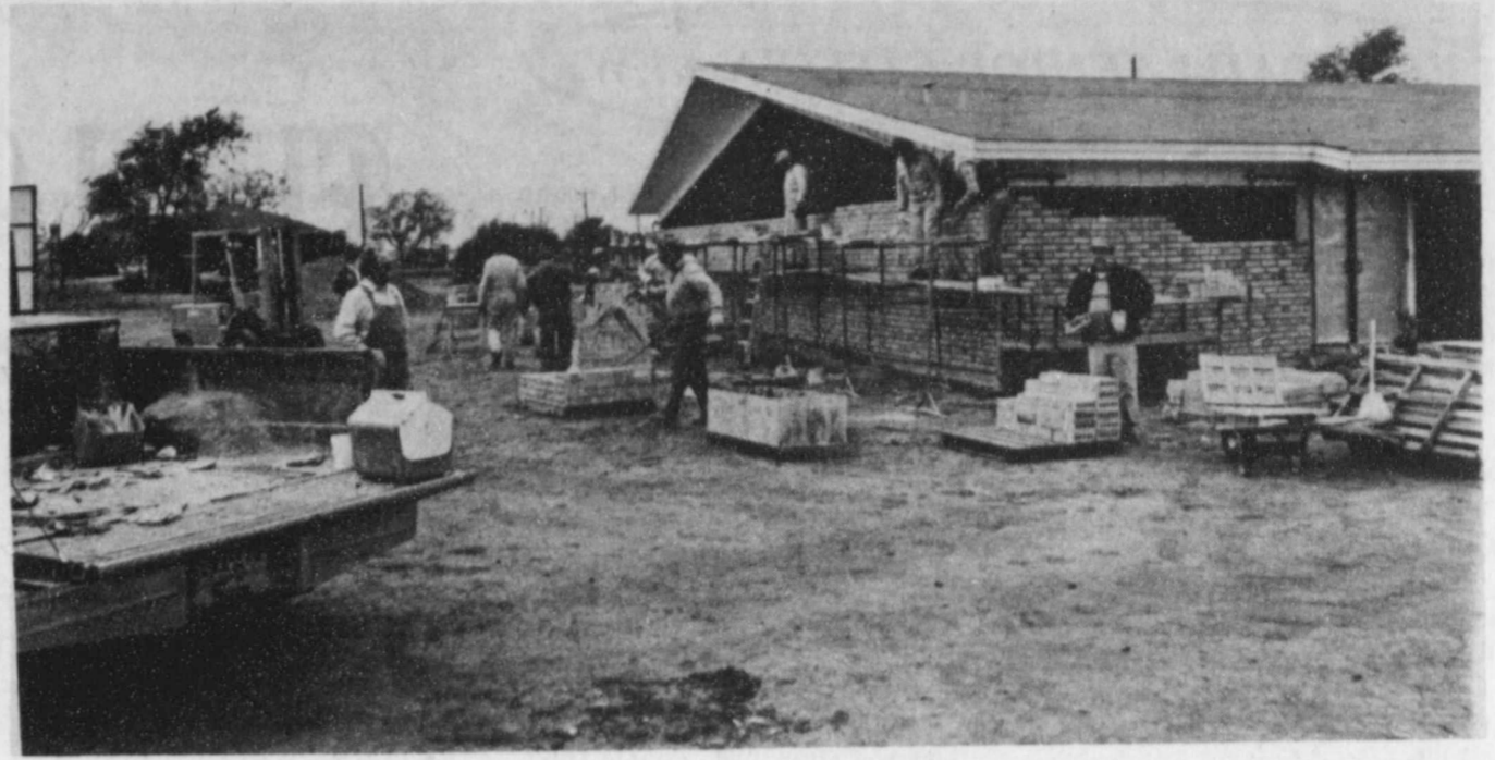
BUILDING A FIRM FOUNDATION —The work has continued on the Mt. Zion Baptist Church which was recently moved to Floydada from the Pansy community in Crosby County. Pansy Baptist Church donated their building and the free labor continues to pour in. Last week brick layers from Pilot Point and Houston re-bricked the structure. Some of the brick had been taken off the building before it was moved and then re-used. Other brick was donated. Brick layers worked on Friday, November 3, from 9:00 a.m.
