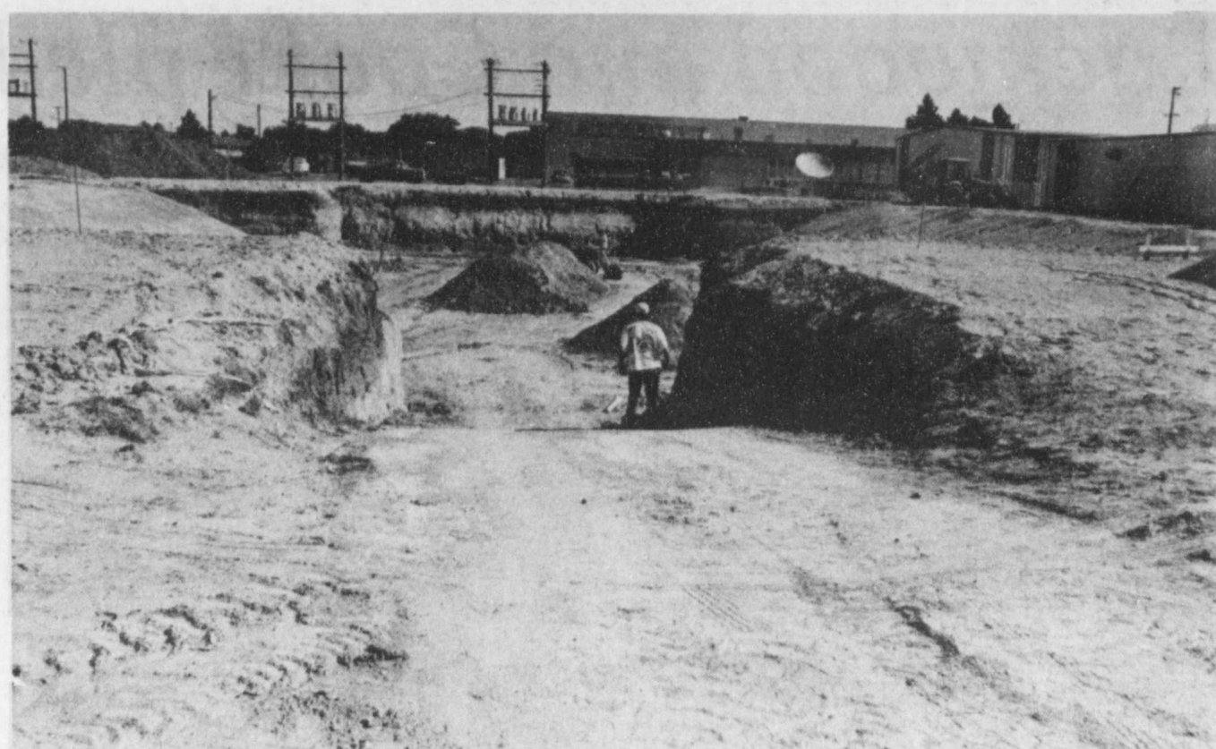
LAYING A SOLID FOUNDATION --Crews have stayed busy throughout the summer getting the ground work ready for the pouring of the foundation of the new Floydada High School gym. The work
