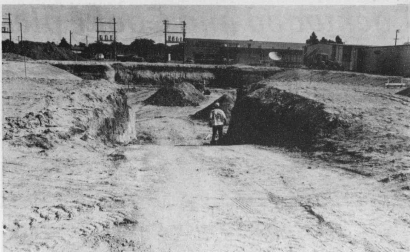
LAYING A SOLID FOUNDATION --Crews have stayed busy throughout the summer getting the ground work ready for the pouring of the foundation of the new Floydada High School gym. The work
