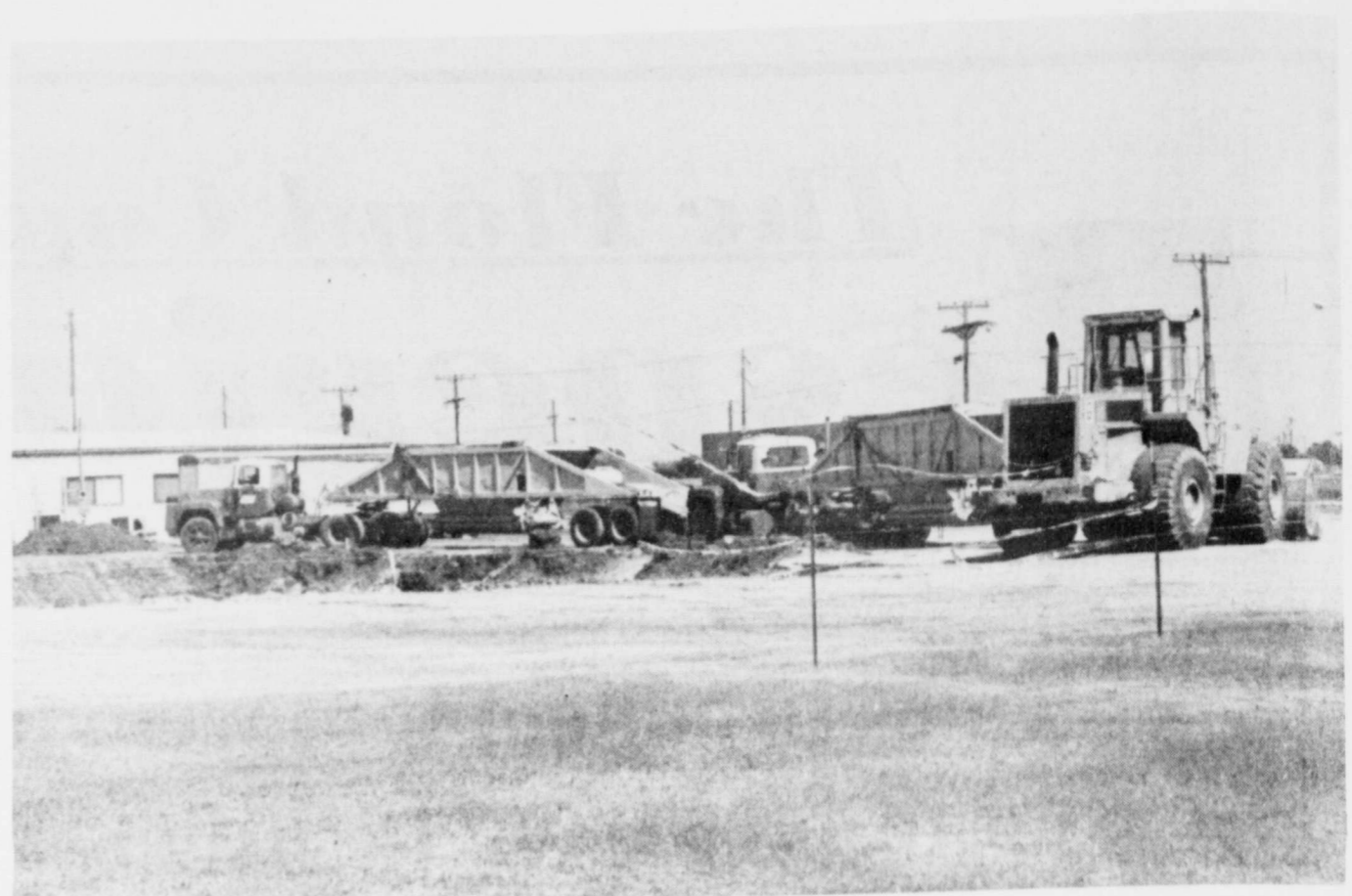
NEW GYM BEGUN -- Work has begun on the construction of the new high school gymnasium at Floydada. The first step is digging the massive hole in the ground to accommodate the facility which will house future basketball events at FHS. The playing
