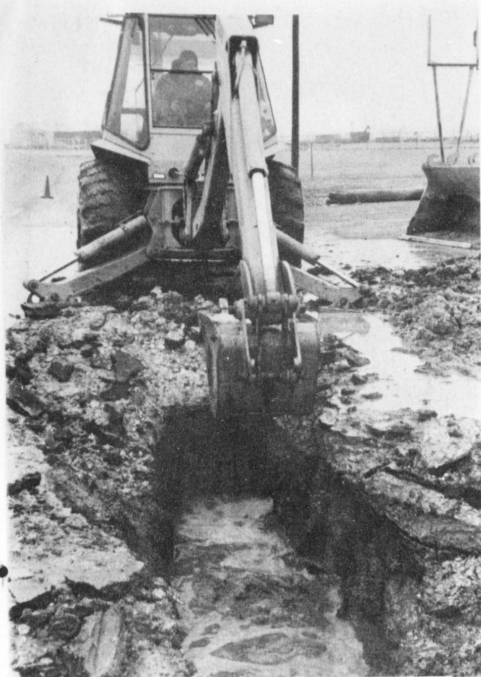
COLD WORK --Floydada city workers battled the bitter cold, Tuesday, after an 8" water main connecting the water tower to the 14" line coming from Lockney, burst. Digging lasted from 9:00 a.m.-3:30 p.m. The city was never without water but did suffer low pressure for a period of time. Staff Photo
