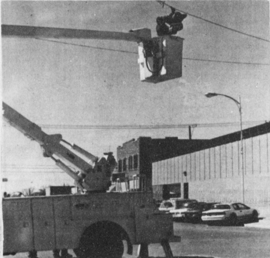
STOPLIGHT CHANGED-- The stoplight at the corner of California and Main Streets in Floydada has been changed to a 4-Way stop. City of Floydada employees installed the new light last Friday --Staff photo
