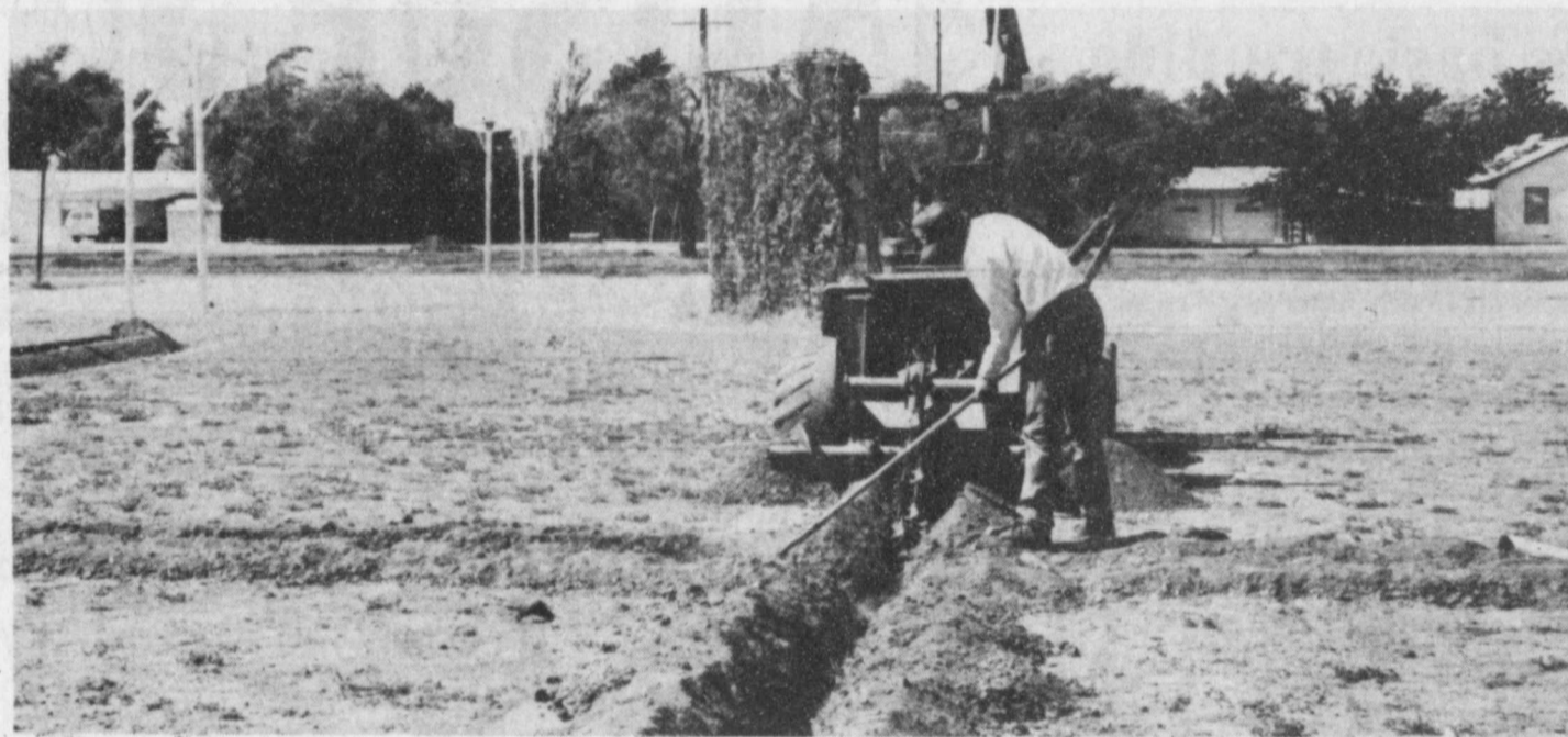
RENOVATING PARK—City employee, Terry Turner, prepares trenches for an underground sprinkler system at Napoleon Park in Floydada. With the help of grant money supplied by Texas Parks & Wildlife the city will be adding playground equipment, picnic tables and other conveniences at the park. Staff Photo
