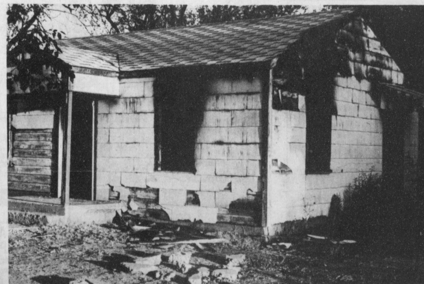
SUSPICIOUS BLAZE--Lockney Police and Fire Marshall are investigating the cause of an early morning blaze Saturday, October 2, at a vacant house in the 300 block of E. Bryant in Lockney. The house was gutted by the fire. Staff Photo
