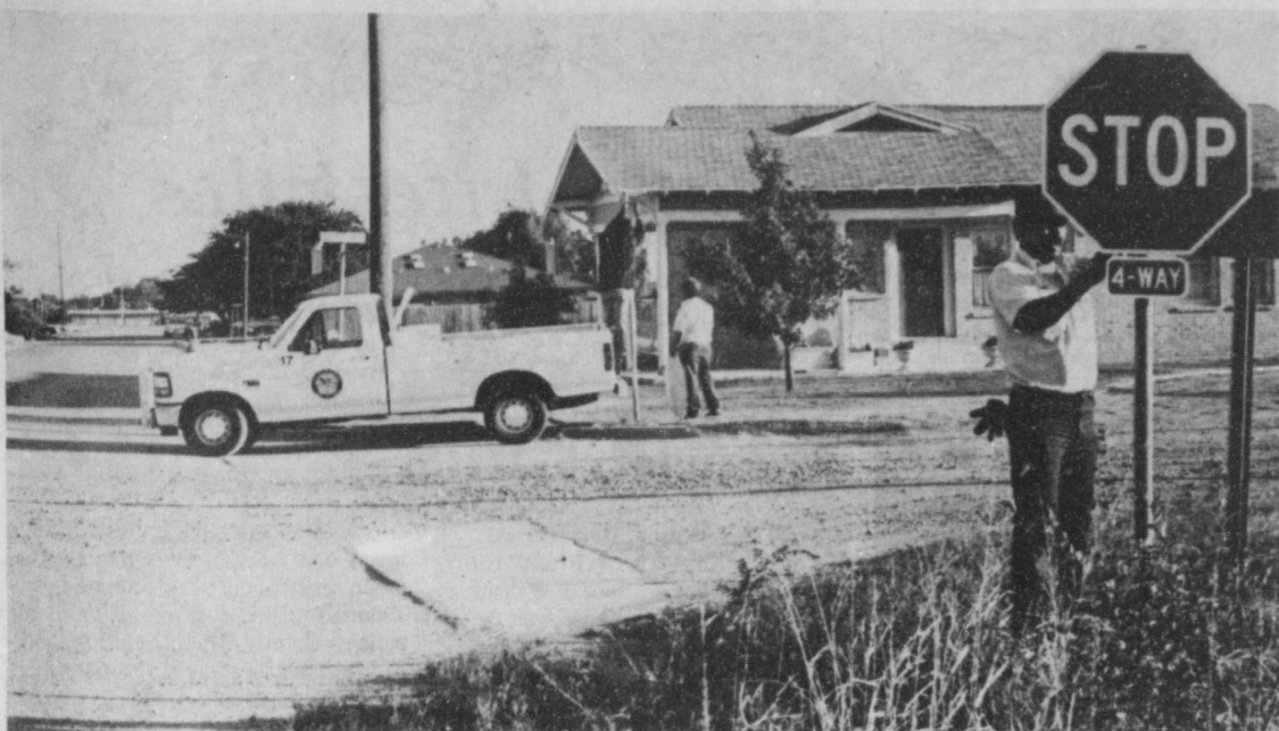
FOUR WAY STOPS -- Two intersections on Ollie Street were the site of early activity on Friday October 1, 1993, as Floydada city workers installed four way stop sign as part of an effort to control excessive speed in a residential area.
