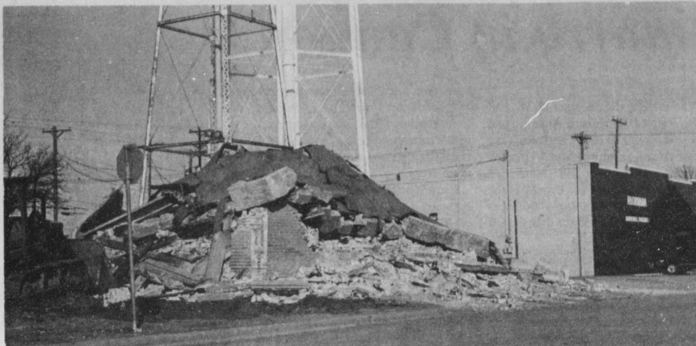
LANDMARK BULLDOZED --The old Floydada Ice House was bulldozed into a heap, on Tuesday, to make way for necessary expansion of City Hall. In order to meet new ADA requirements City Hall will be adding new and easily accessible bathrooms on to the current structure. More room for record keeping will also be added. Staff Photo
