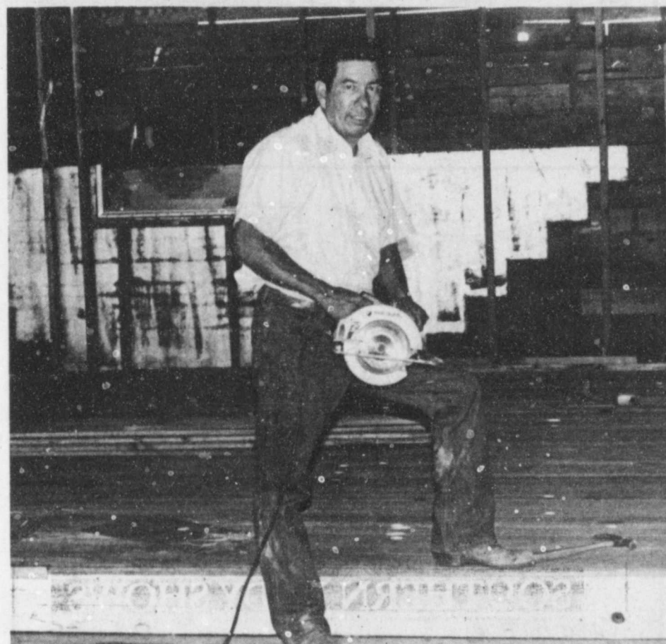
BUILDING PROJECT CONTINUES —Rev. Rendon, along with his congregation, continues to work on the church which is being built on north Main Street in Lockney. According to Rev. Rendon, "We are grateful for the donations we have received. People have been generous." Staff Photo
