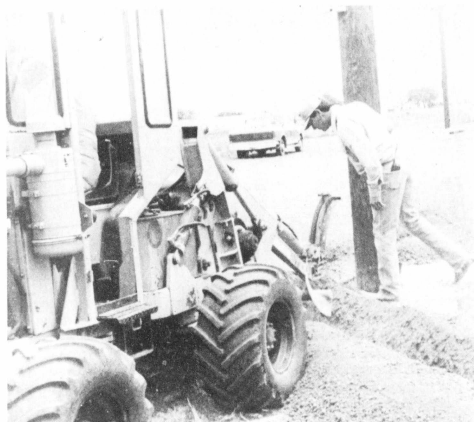
LIGHTS ARE GOING UP —Workers began installing the lights at the Little League baseball park in Lockney. When sign-up was over there were more games scheduled than could be played in daylight hours due to the number of kids signed up for T-Ball and Little League. These lights were made possible through a city wide fund raising effort. —Staff Photo
