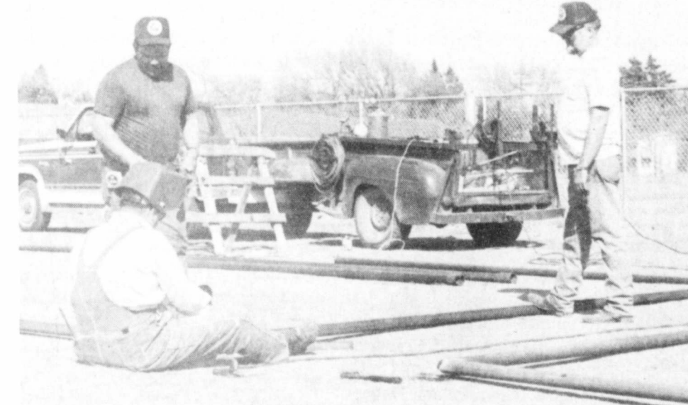
JOINT EFFORT -- Jimmy Collins (in welding helmet) is assisted by Jesse Morales (left) and City Manager Gary Brown (right) in assembling a steel framework. The framework is for the new 'bull pen' area of the refurbished baseball facility at Floydada City Park. —Staff Photo
