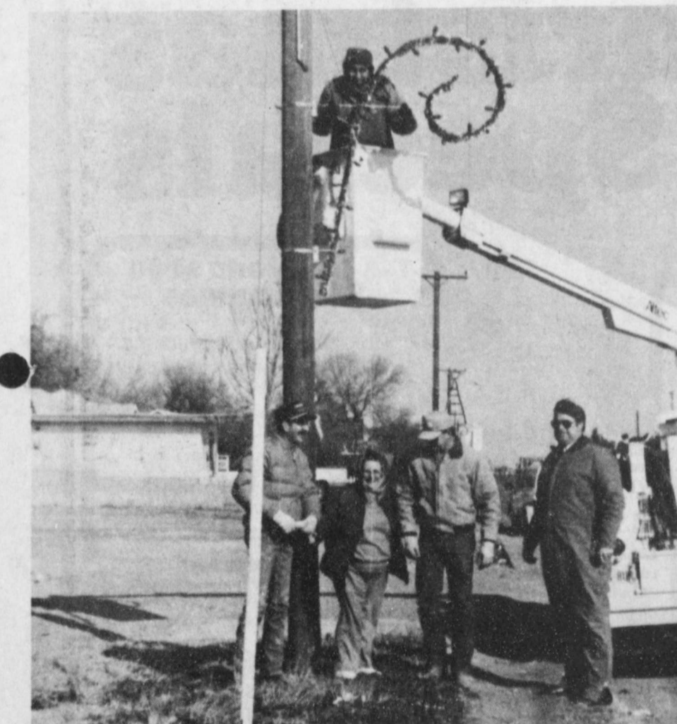
CHRISTMAS LIGHTS INSTALLED—Robert Webb braved the cold and wind to plug in the new lighted Christmas ornaments on Main Street in Lockney on Monday, December 2. Helpers (?) on the ground included Bill Davis, Vera Jo Bybee, Bil Anderson and Jim Bob Martin. Staff Photo
