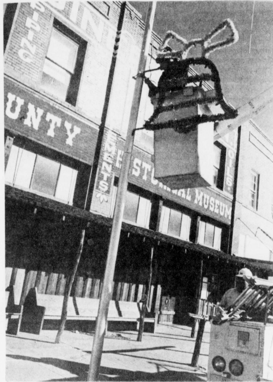
DECK THE HALLS—City workers took advantage of mild temperatures on Monday, to install Christmas decorations around the city of Floydada. The yearly Santa labor is supplied by Floydada Power and Light, SPS and Light-house Electric. Shown in the bucket, struggling against winds and not enough hands is city employee David Rodriguez. Jesse Morales is on the ground.
