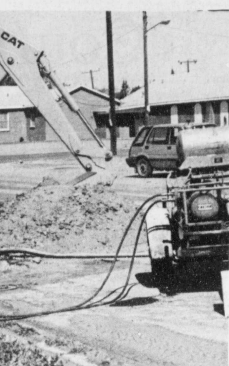
WATER MAIN BREAKS — Floydada city workers scrambled to repair a broken water main on Grover Street near Second Street on Monday, April 29. The crews worked diligently to dig out the problem area, pump out the water and install new lines in order to restore water service to areas of the city which were without water due to the break. Staff Photo
