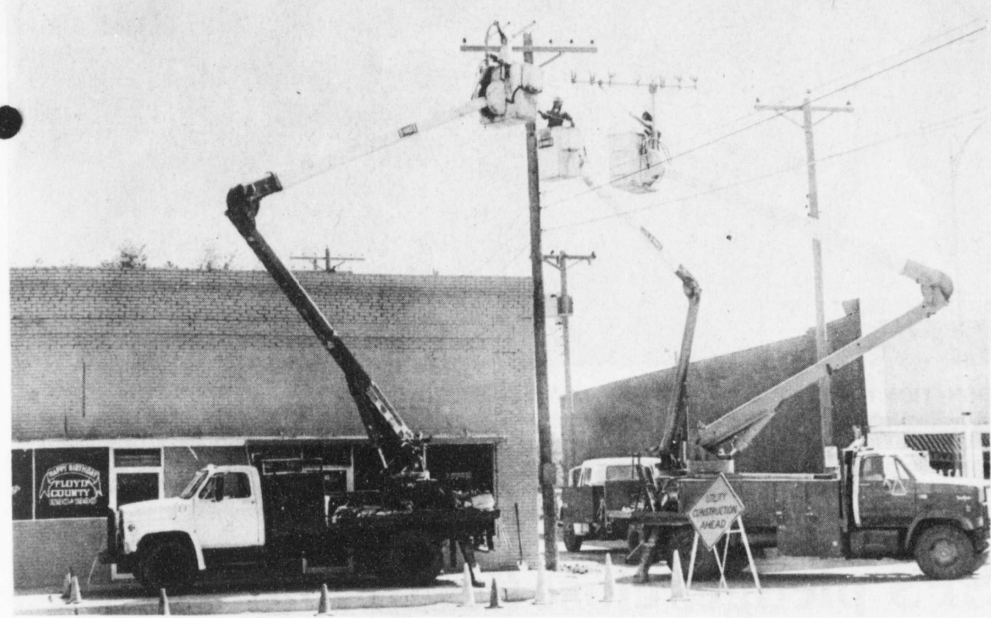
DISTRIBUTION LINES BEING REPLACED — These three trucks with buckets lifted into the air are becoming a regular sight around Floydada as workers from K & C Construction of Midland, Texas, move about the city replacing electric distribution lines which are more than fifty years old. The work is part of a multi-year on-going project to see that Floydada Power & Light continues to be a viable electric distribution facility. Staff Photo
