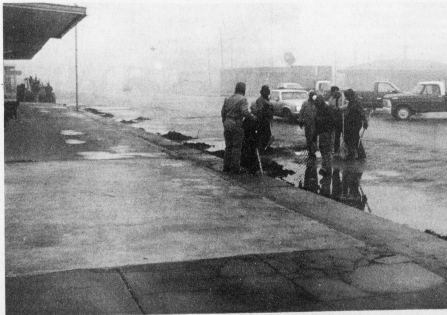
FOG SHROUDED CLEANUP — As fog filtered through the streets of Floydada, so did a swarm of workers from local gin facilities last Wednesday, January 9. The busy bundled up fellows were on a mission to remove any street
