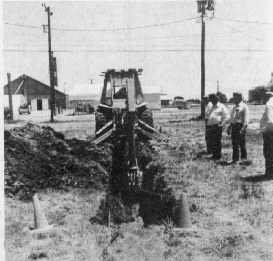
BUILDING THE OVEN--The City of Floydada provided a backhoe on Tuesday, to dig the hole that will be used to hold the mesquite wood grubbed off the caprock and the bar-b-que for the noon meal on Saturday. Staff Photo
