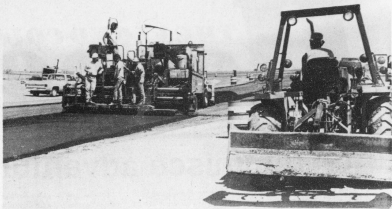
PAVING EQUIPMENT of Duinick Brothers is shown in the final stages of the $2 million-plus paving and improvements on Highway 70 east of Floydada. According to Shelby Peoples of the Lubbock office of Texas Department of Highways and Public Transportation, the project has
