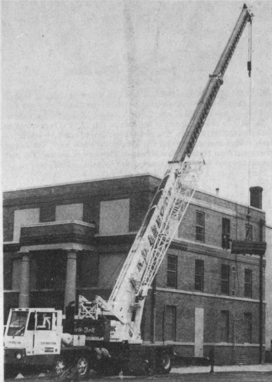
EASY DOES IT —Equipment had to be brought through a window to the third floor of the Floyd County Jail during renovation started on Friday. Cranes lifted bunk beds and bars to the floor that will be remodeled to fit the specifications of the Texas Jail Standards. Fourteen bunks are being added to the third floor along with showers and lavatories. The detoxification room is also being remodeled into a holding cell. —Staff photo
