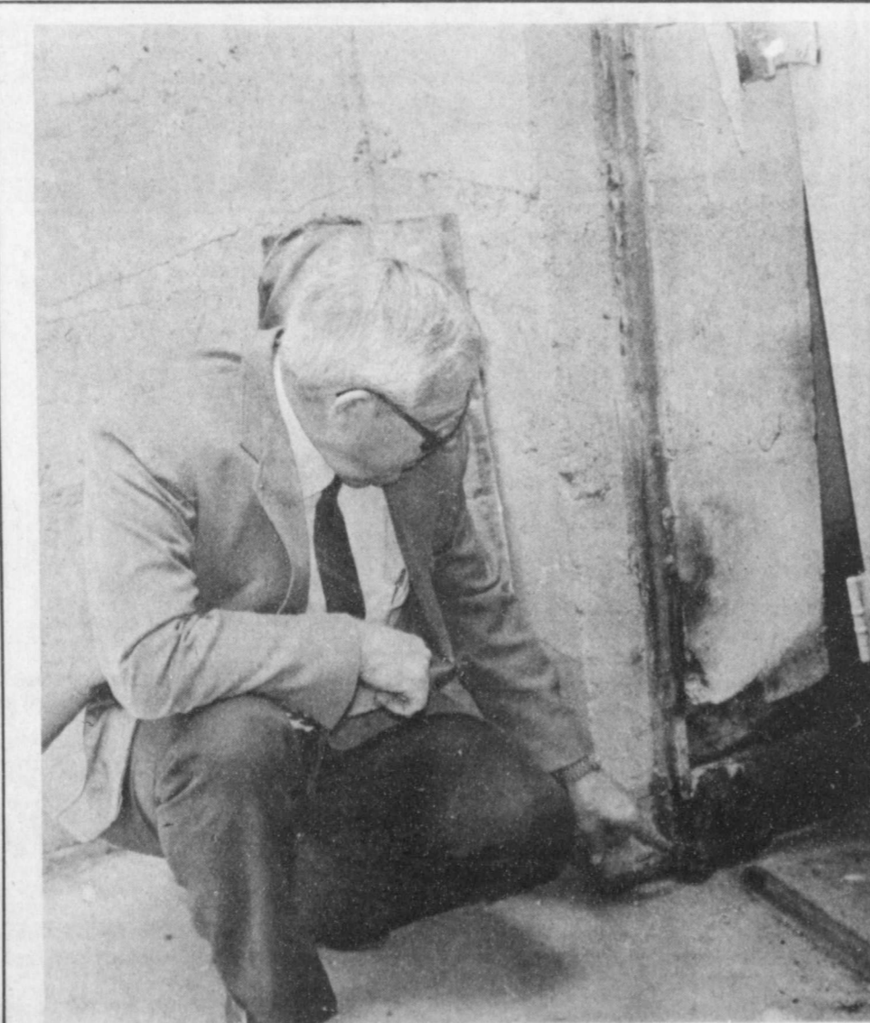
IT STARTED HERE — Charles Tyer, principal of R.C. Andrews Elementary School, points to wooden framing for a metal door where a Sunday fire started. Damage estimates were not available at press time, but the blaze was confined to a single storage room. — Staff photo
