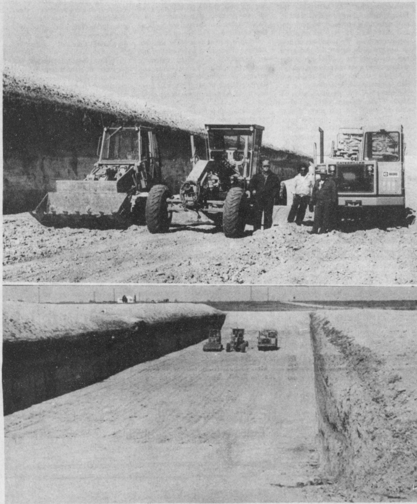
LANDFILL BEING DUG —Three machines and operators [left to right] Bill Hopper, Manuel Reyes and Benny Martinez are shown digging out "the last hole dug in the original dumpground site," according to Hopper, who along with Martinez are employed by Precinct Four. Reyes is a City of Floydada employee. The city and county are cooperating in the project to dig the 66 feet wide, "about 300 yards long" and 24-25 feet deep pit. Machinery being used are a
