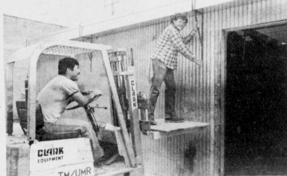
CHAMBER PROJECT CONTINUES—Blanco Offset Printing has installed a new metal guttering to carry rainwater off the roof of the business. Also contributing to this local clean up, fix up endeavor were Hammond Sheet Metal where the guttering was made, and Russell Equipment who fabricated the braces. Blanco employees Juan Martinez and Jim Huggins urge other Floydada businesses and residents to join the Chamber of Commerce project in an effort to make Floydada a beautiful place to be during the 1986 Texas Sesquicentennial Celebration.
