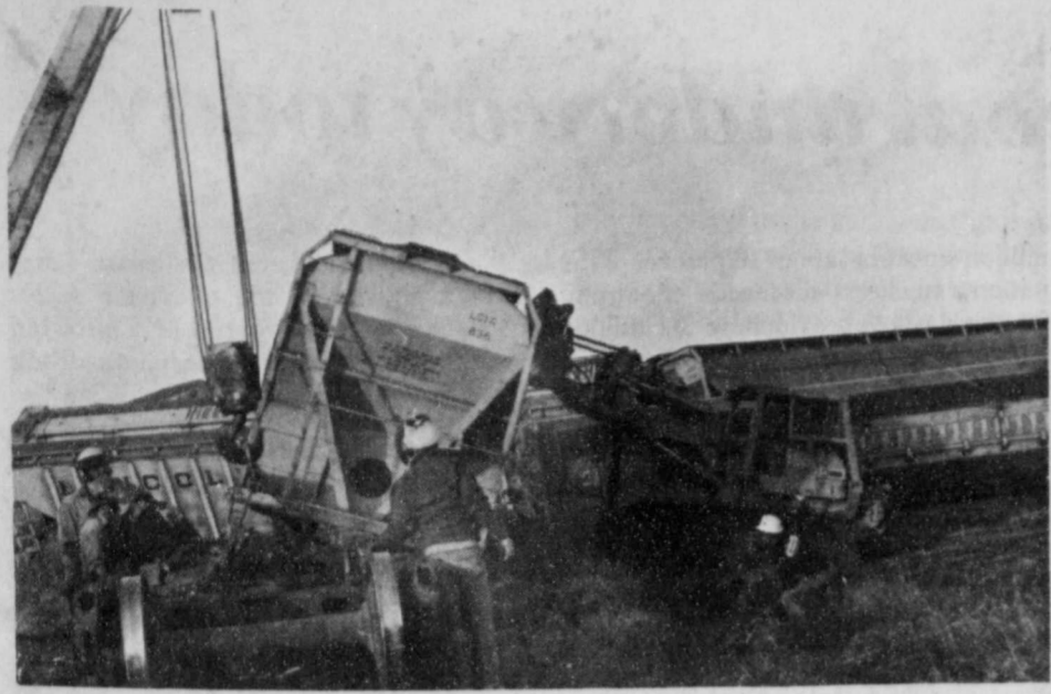
SEVERAL MEN and pieces of heavy equipment were required to set things right following a derailment near South Plains last Saturday.
