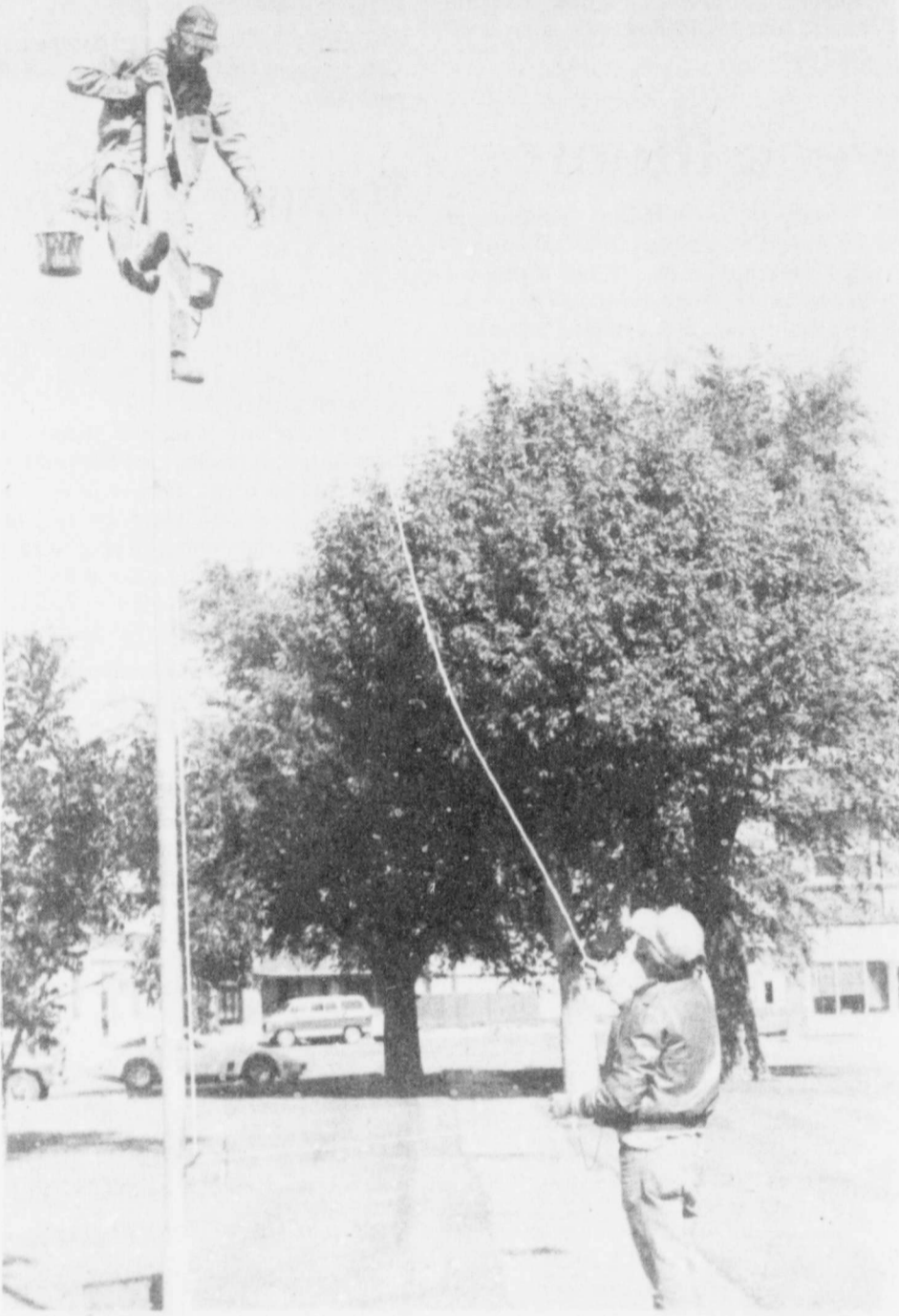
STEEPLE JACK AT WORK - Bob Teague guides the ropes as Phil Baasch shinies up the flagpole at the Floyd County Courthouse. The pair are from Steeple Jack Service in Selma, California and they make the circuit every three or four years to paint poles in eleven western states. Says Bob, "A pole like this costs about $130.00 to paint if it is in good condition." The highest pole they have done is in Calapatia, California and is 184 feet tall. The Floyd County pole is about 30 feet tall.
