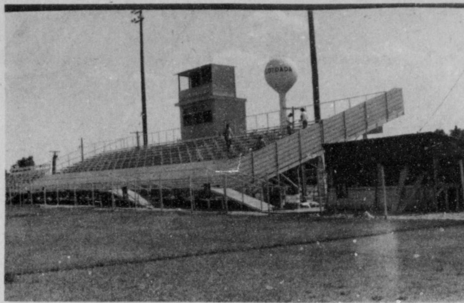
NEW ALUMINUM BLEACHERS —Installation of new aluminum bleacher seats at Wester Field is advancing at a steady clip. The press box has been covered with siding and the home side will have a whole new look this fall.
