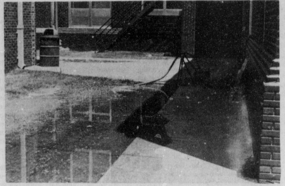
JUNIOR HIGH WATER LEAK —Shown above is one of the five pumps used to remove water from the lower areas of the junior high last week after a rusted fitting flooded the auditorium.
