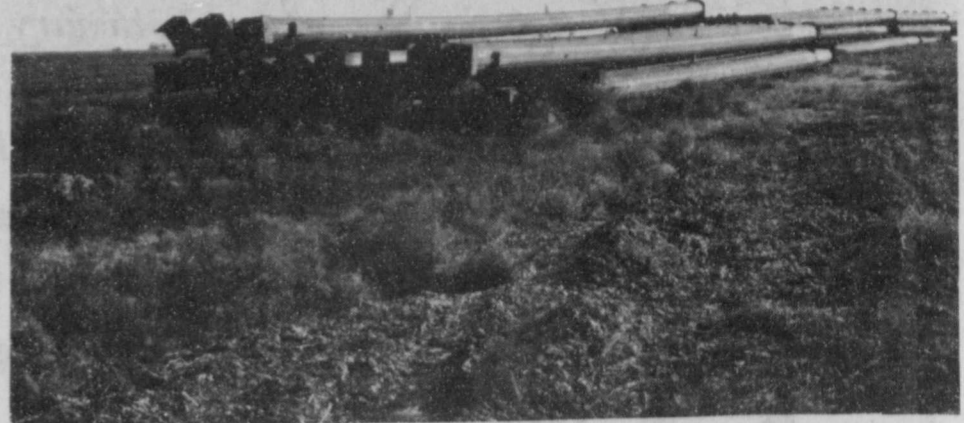
SOUTHWESTERN PUBLIC SERVICE poles are being delivered to a distribution point on Highway 70, just north of Floydada. Construction in this area will not start until contractors make their way from Paducah.
