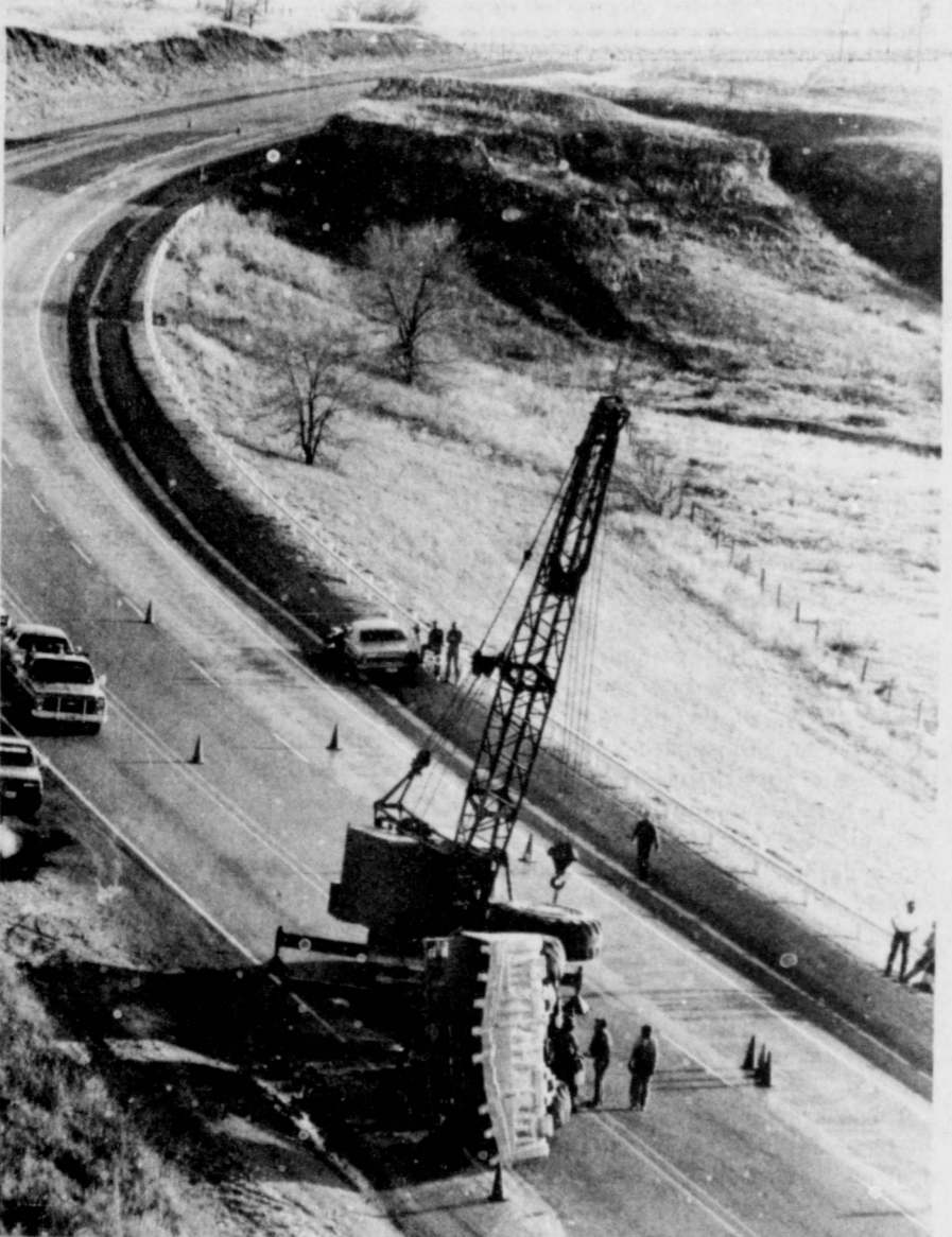
THE CRANE has lifted the loader to its side after it turned over in the steep grade in Blanco Canyon.
