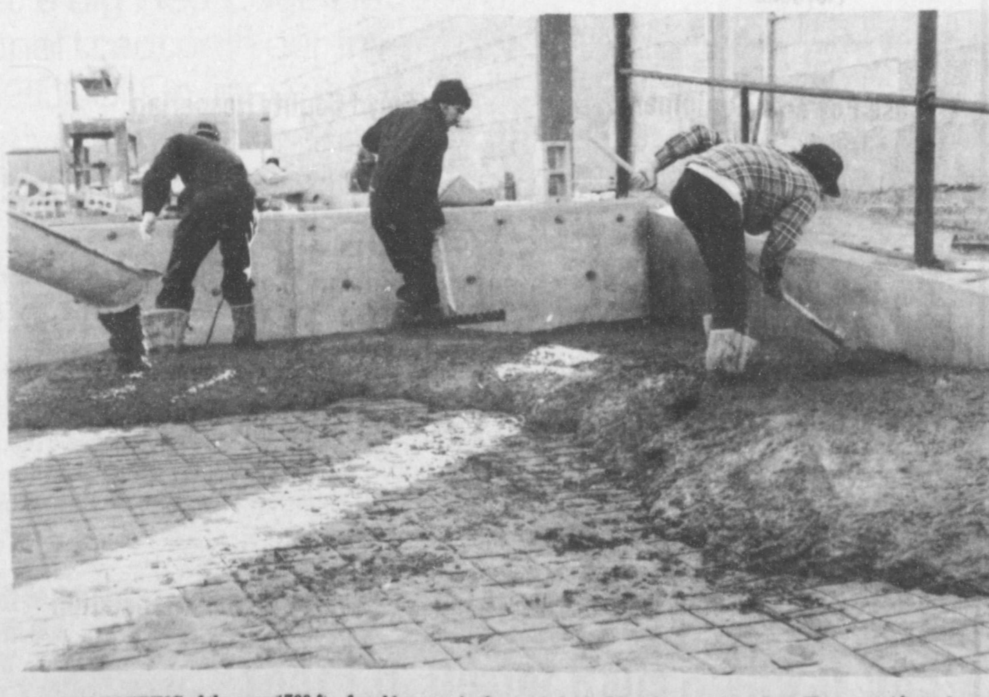
CEMENT POURING of the over 1700 ft. of parking area in the new post office began Wednesday morning. Completion date on the building is set at April first. The cement is made on site in the portable plant.
