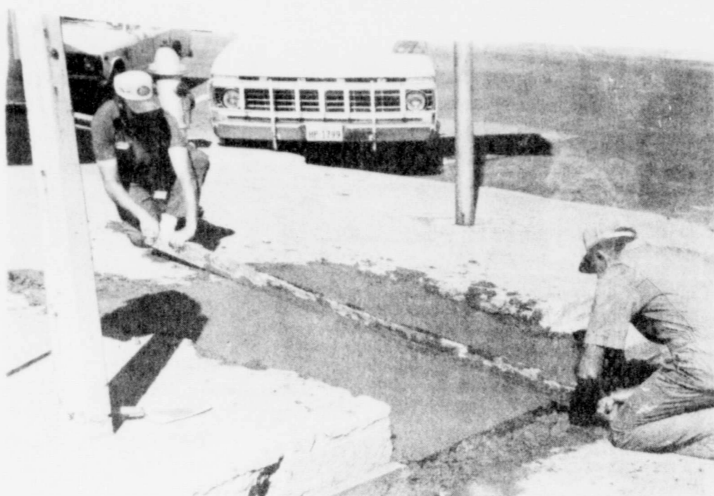
TED JORDAN AND BOB COPELAND are forming the cement in front of Thompson's Pharmacy.
