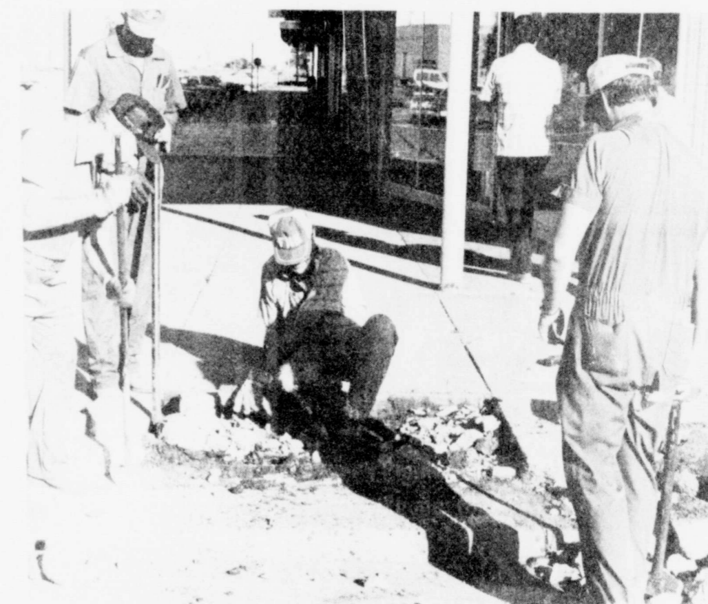
LIONS STARTED BUSTING CONCRETE Thursday. Left to right—Aldine Williams, Bob Alldredge, Gary Brown, Ted Jordan in front of Arwine's Drug Store.
