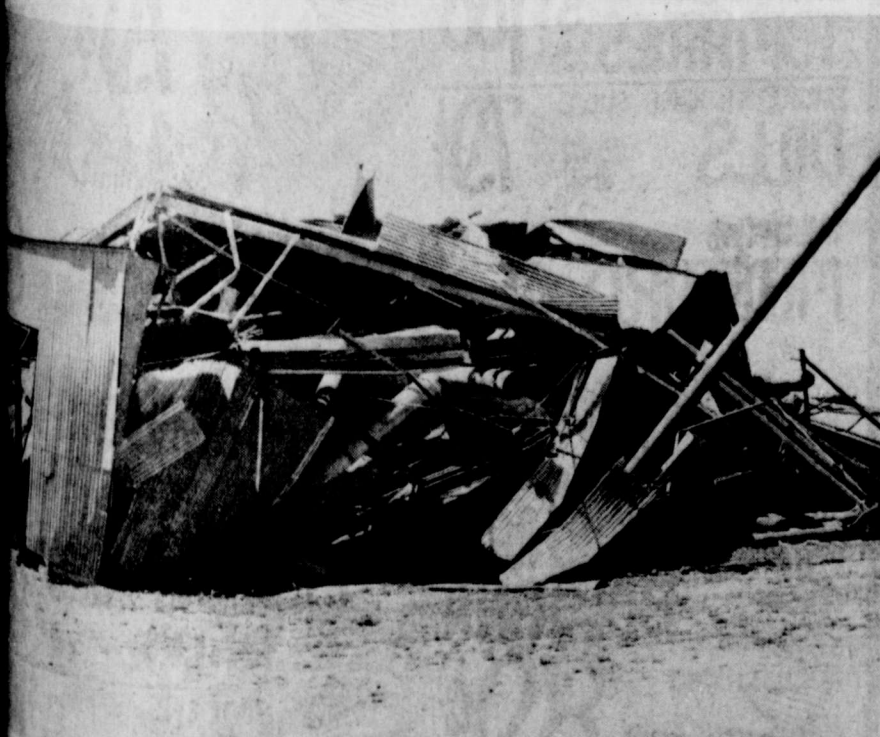
GIN didn't explode from pressure. The wind hit a side wall pushing it 10 feet. The roof collapsed without support. New equipment had been recently installed and the building remodeled. See Farm Page for other pictures of the gin.
