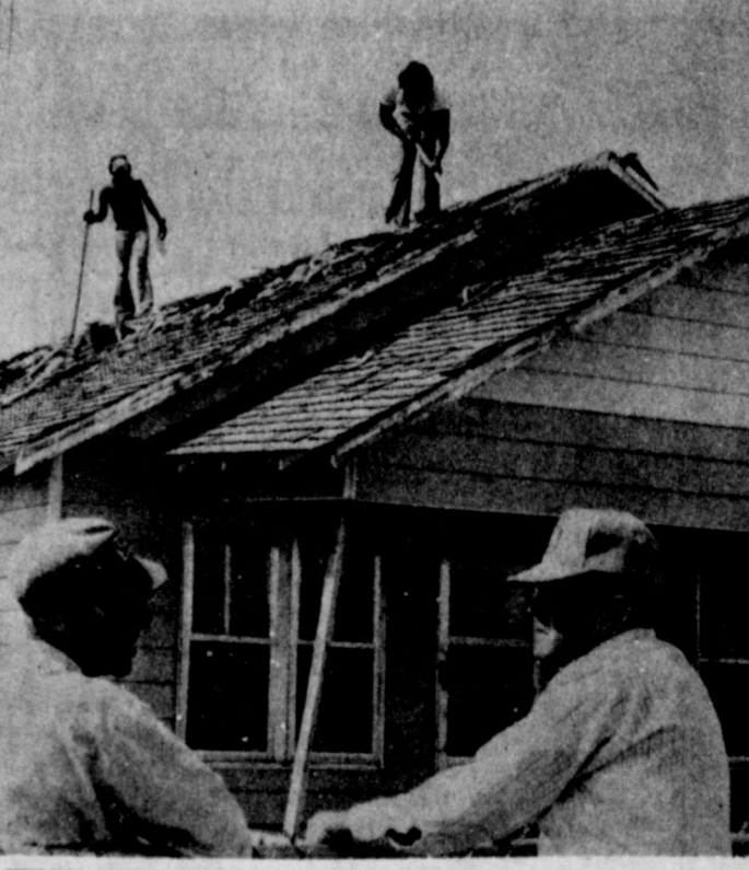
FIRST RENOVATION. Andrew Reyna and Dorris Blasingame talk over details of Reyna's home remodeling under the city's rehabilitation plan. The house at 516 East California is to get a new roof, new cement porch, attic insulation and wall heater.
